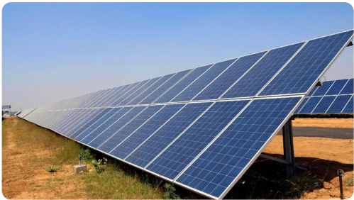
Solar power plant (IANS)
